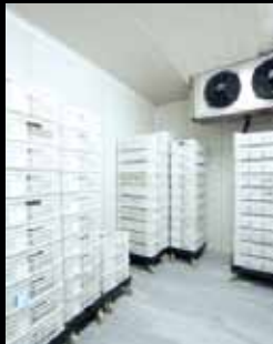
Walk In Freezers
